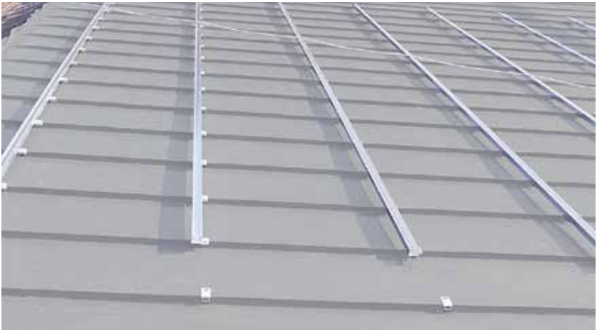
Elpo | Neumarkt - Italy System: 39,60 kW | Seam metal with S5!
